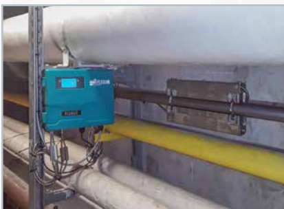
Measuring point with a stationary FLUXUS® G721CA transmitter and the ultrasonic transducers mounted in Variofix L rails on the pipe.
